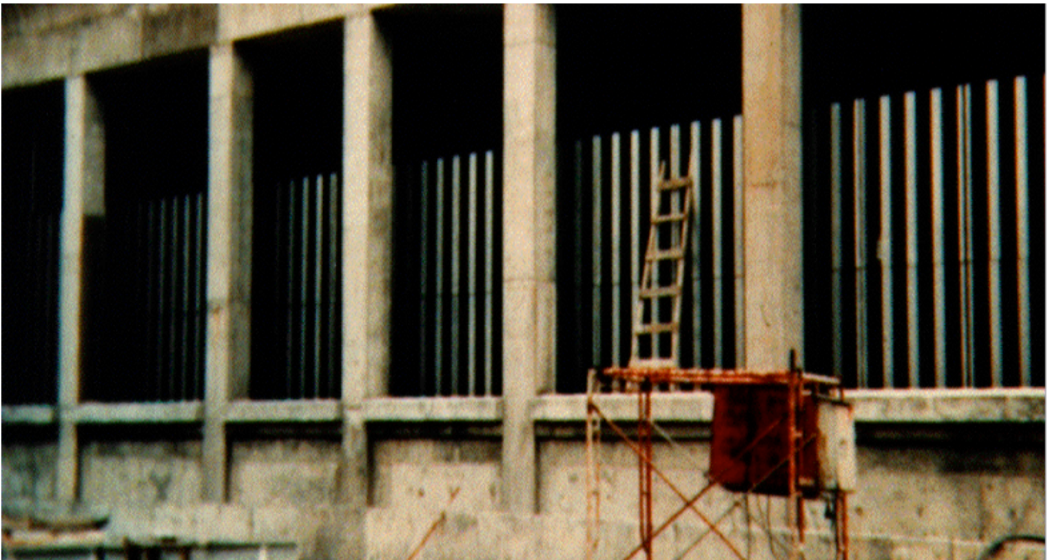
Taipei underground railway - 19m width x 4.5m height, consists of 45 modules sound attenuators installed in concrete tunnel shaft
